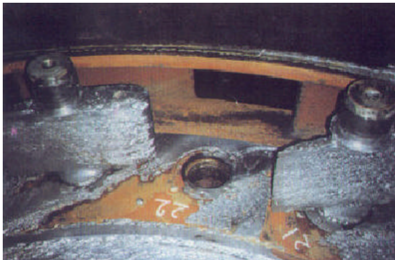
Figure 4 Severe erosion on Francis Turbine ring and wicket gate
