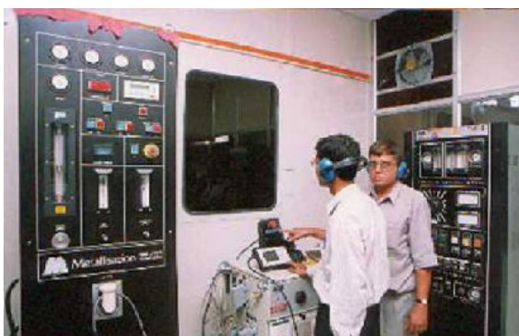
Figure 5 BHEL's spray control room
