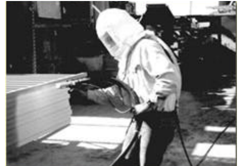
Hand spraying Zinc for corrosion protection using electric arc equipment. (photo courtesy of Thermion U.S.)
